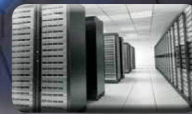
UPS & Data Centre
