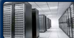
UPS & DATA CENTER
