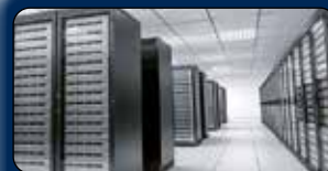
UPS & DATA CENTER
